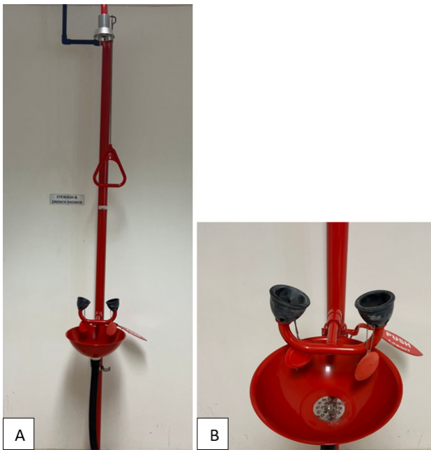
Figure 1: A): Complete eye wash assembly; B): Eye wash station
